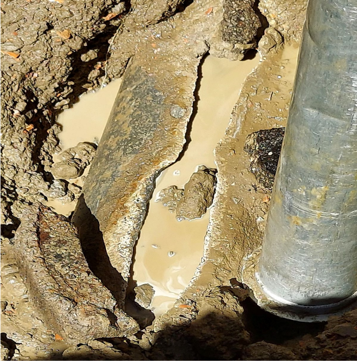
PICTURE 1: Exposed pipe with top gone.
